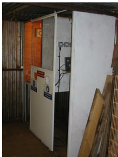
battery charging station
