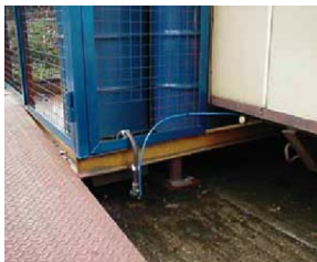
Bund pump innovation
