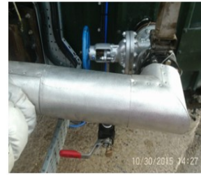
Modern system with a bleed valve which would confirm effective isolation of the pipeline
