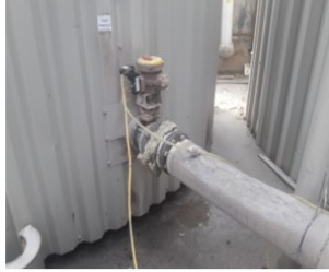
Actuator valve; with no physical way of knowing if isolated effectively
