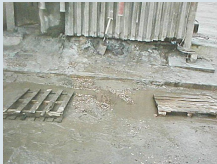
An untidy customer site: Slips, trips and falls are the most common cause of injury to drivers on customer sites.
