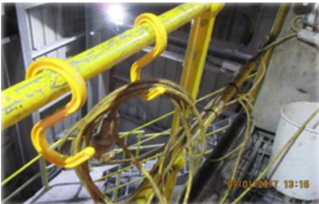
S Hooks for keeping cables clear of walkways
