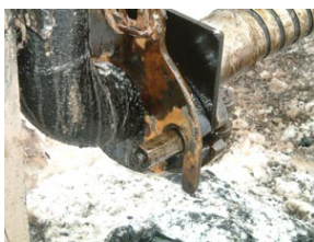
Modified flange for bitumen delivery
