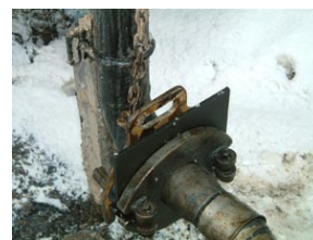
Modified flange for bitumen delivery
