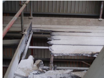
Burnt Scaffolding Boards
