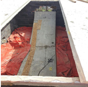
Fig. 1 - Damaged slab on ground
