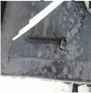
Bar used to by-pass system
