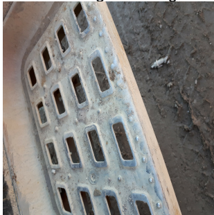
Footplate in poor condition
