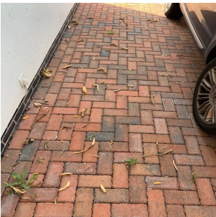
Debris in drive
