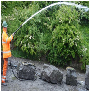
Picture 2: Pump Working
