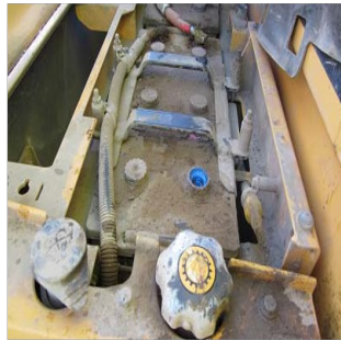
ATD Battery with Cap Missing
