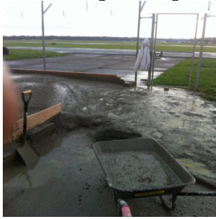
Spillage when wall collapsed
