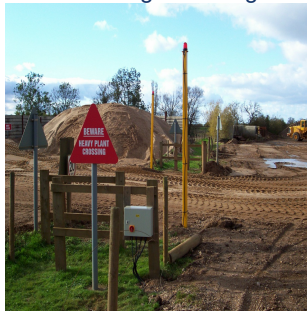
Public footpath flashing light system
