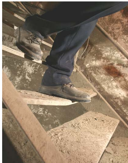
Worn stair treads lead to slips, trips and falls.
