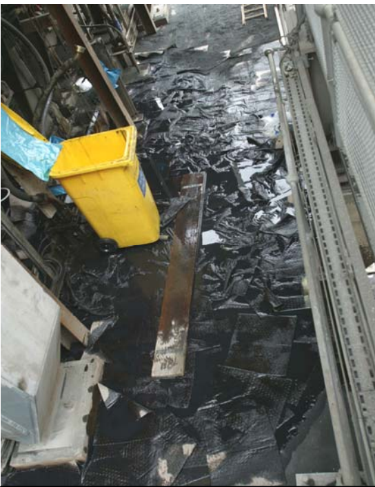
Oil spill and badly maintained walkway.
