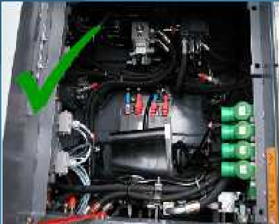
Compartment showing components
