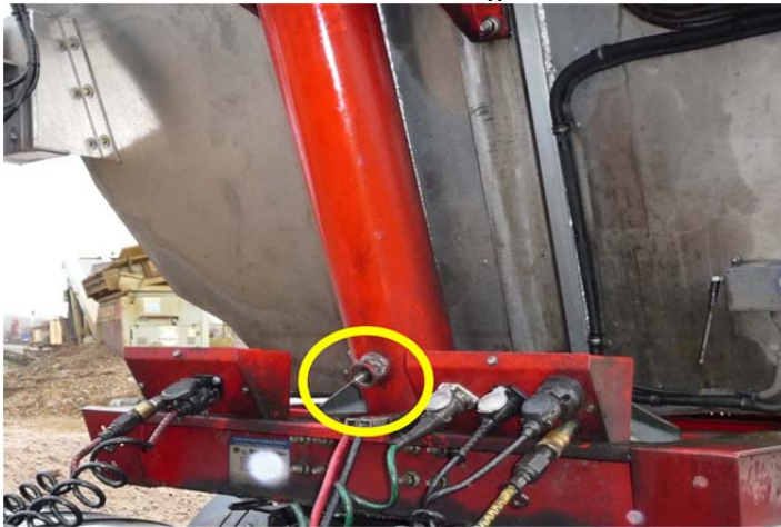
Housing where the valve was connected
